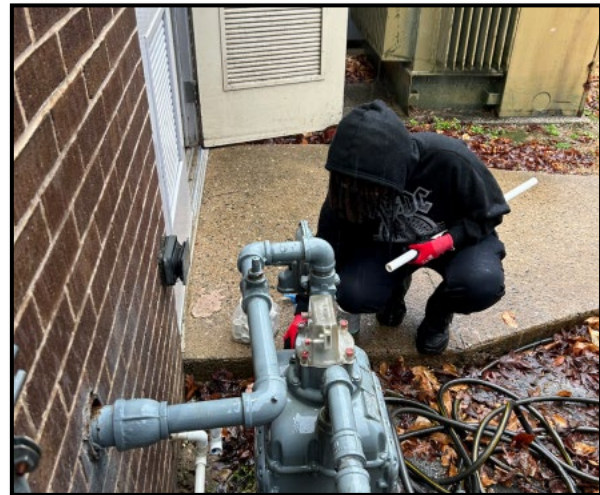
Leelaje Mullings, WJCC student, HVAC Intern, gaining experience in HVAC systems.
