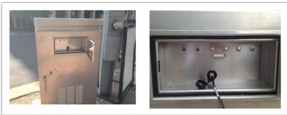
Flasher Data Port: A dedicated hardwire connection to the County network at traffic signal cabinets
