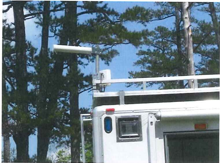
Figure 2- Network Equipment Mount at Foxfield Races
